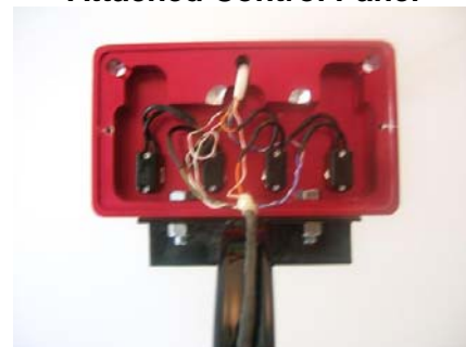
Attached Control Panel
