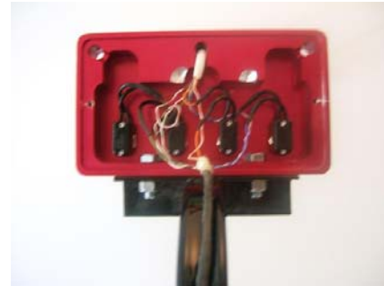
Attached Control Panel
